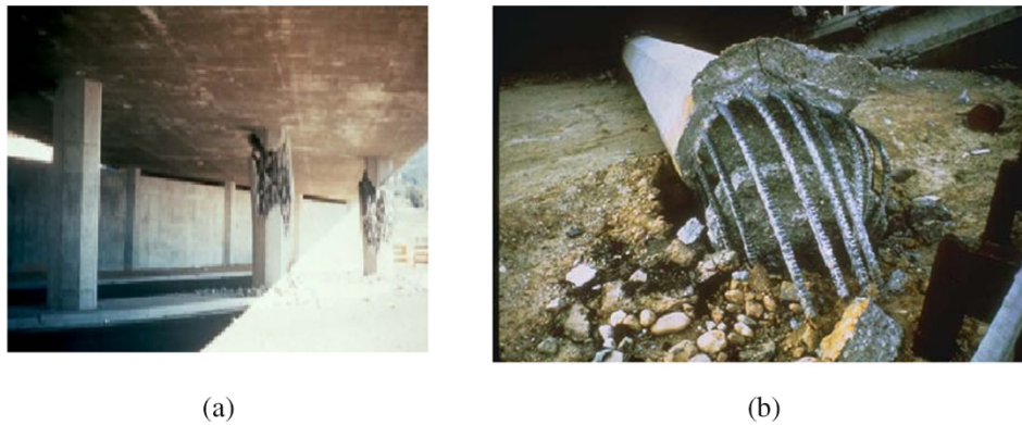
Fig. 1. Bridge column with (a) shear failure and (b) pull-out failure in 1971 San Fernando earthquake [39].
